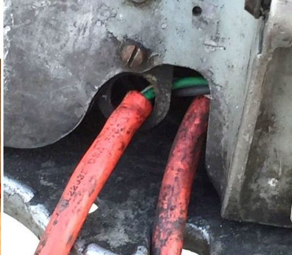
Damanger connection to power machine.
